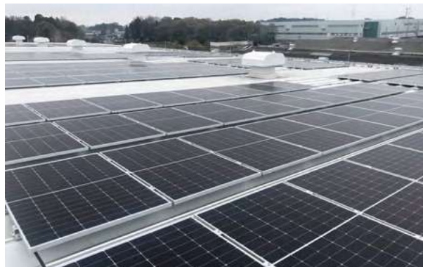
Solar panels at Itoki All Steel Co., Ltd.
